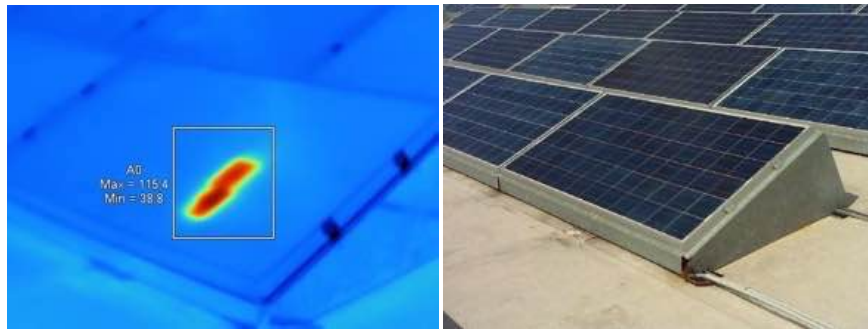
Figure 5. Defect in a solar panel
